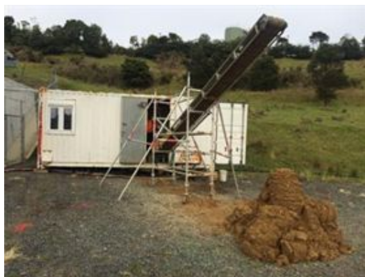
Portable Centrifuge in operation, Ardmore WTP
